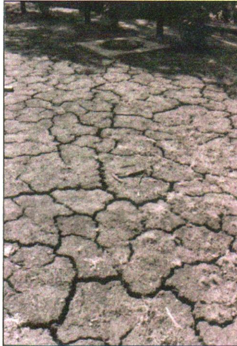
Figure 1: Polygonal pattern of surface cracks in the dry season. These cracks are approximately one inch wide at the top. Note sewer manhole in background.
